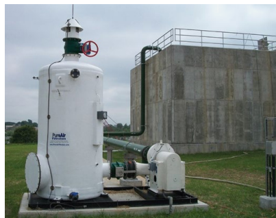
VERTICAL BED SCRUBBER
