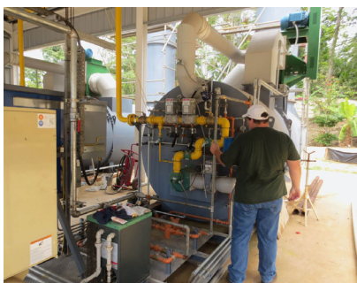
125 GAL/HR LIQUID WASTE THERMAL PLANT
